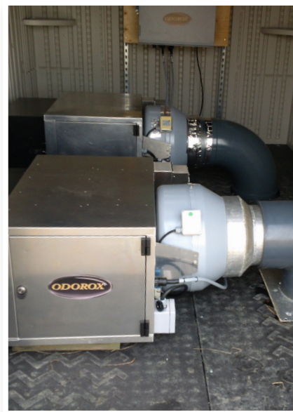
Hydroxyl generators installed on the upper vault.
